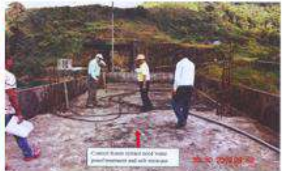
Damaged Control Room Terrace
