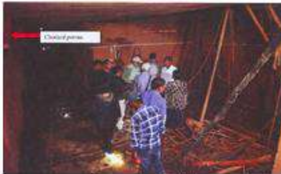
Porous pipe choked
