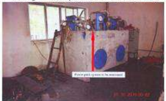
Damaged Power Pack System
