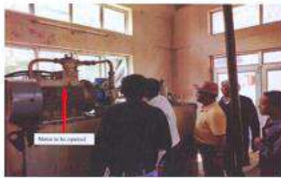
Damaged Motor of Radial Gate No.5
