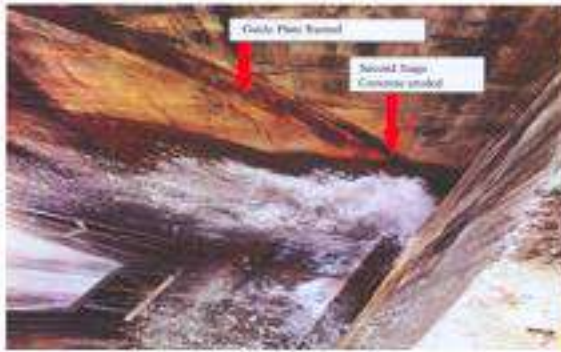
Radial Gate Guide Plate & Second Stage Concrete Eroded
