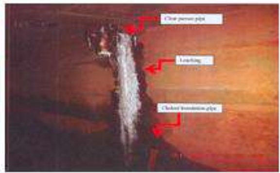
Leaching inside the dam Gallery, Foundation pipe choked
