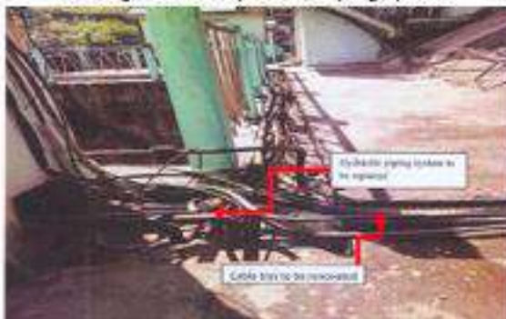
Damaged Hydraulic Piping system and Cable Tray
