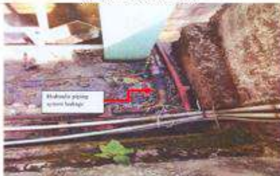
Leakages in the Hydraulic Piping system
