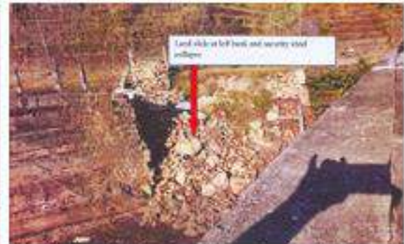
Landslide at Left Bank and Security Shed Collapsed
