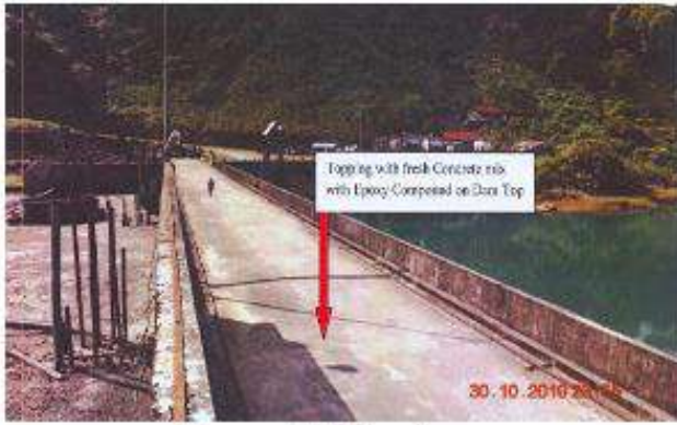
Damaged of Dam Top
