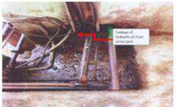
Leakages in the Hydraulic oil from Power Pack
