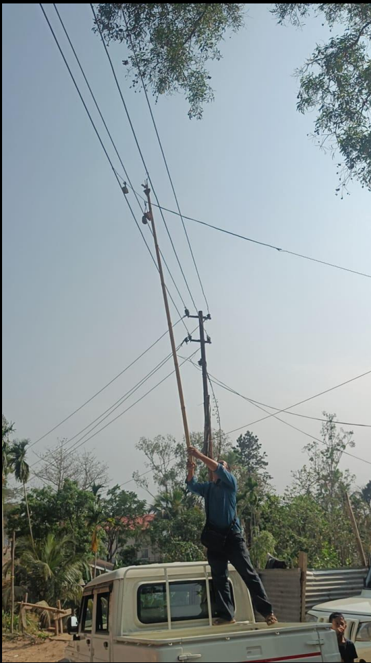
De-hooking/ disconnection of illegal hooking
